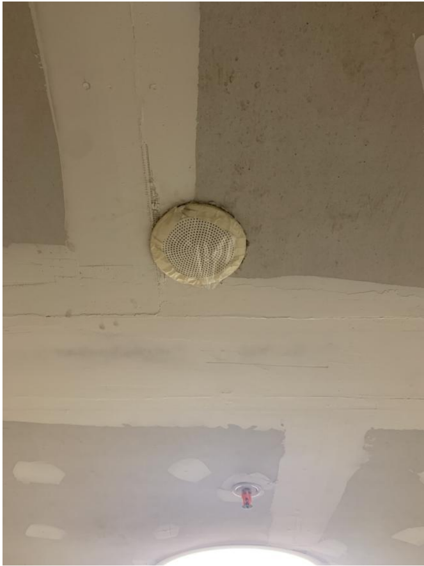
PA system corridor Tower-B
